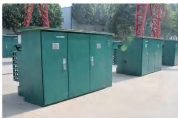
光伏/风电组合变压器 Photovoltaic / wind power combined transformer
