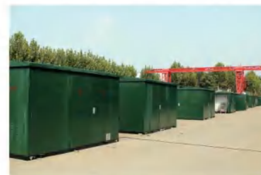
神华箱变 Shenhua box type substation
