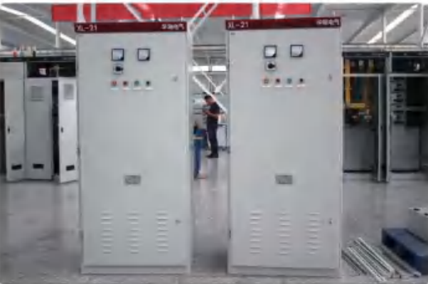
XL 动力配电箱 XL power distribution box
